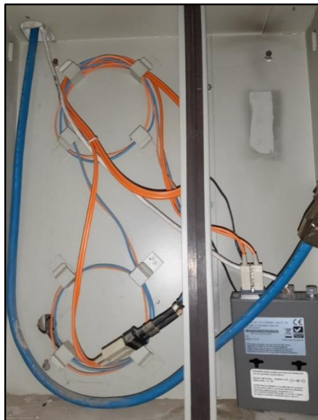
Figura 5. Gabinete de media converter.
