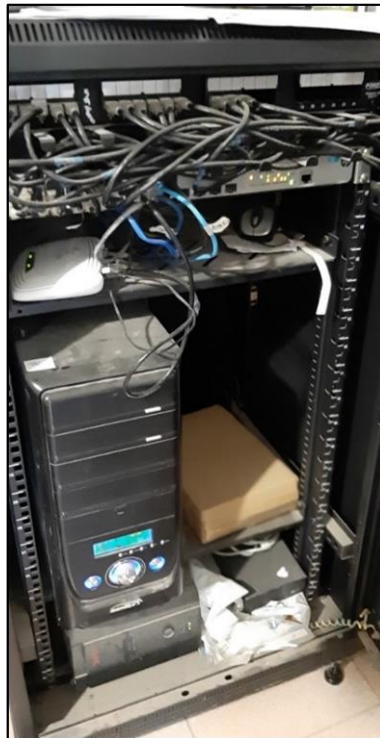
Figura 8. Rack principal del sector de OAT.
