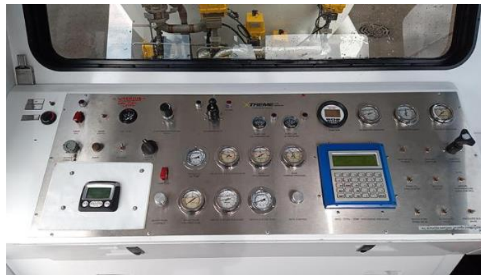
Figura N°66: Tablero de control. https://www.google.com/imgres?imgurl=http://rigsmarket.com/wp-content/uploads/2015/11/20151005_111021.jpg?v%3D1638146257&tbid=qc8OjllqdF3rdM&vet=1&imgrefurl=http://rigsmarket.com/main/nitrogen-equipment/nitrogen-840k-direct-fire-automated/&docid=R0vYFXnV9ugRYM&w=640&h=360&hl=es-US&source=sh/x/im#imgrc=qc8OjllqdF3rdM&imgdii=wTKsHWzOyzK3M
