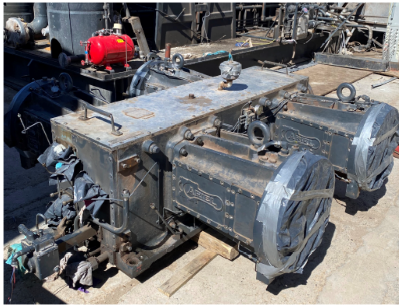
Figura 5. Compresor Ariel JGK4.
